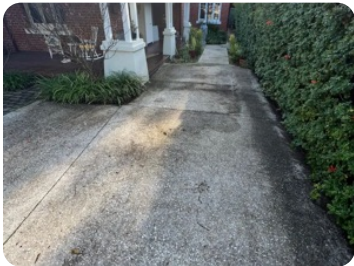
01 Exposed aggregate, before Traffic film and organic growth.
